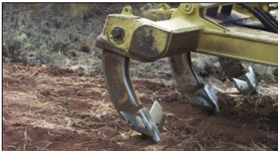
Figure 38—Larger equipment is used for deeper ripping to increase infiltration and break through water repellent soils.
