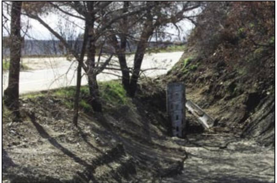
Figure 91—Riser located next to county road and receives frequent maintenance to remove material.
