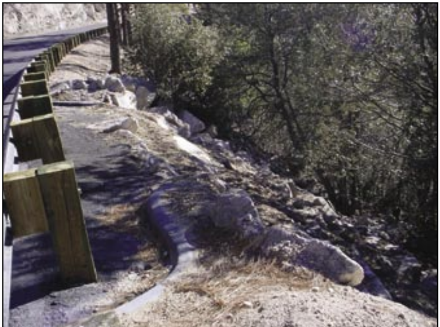
Figure 73—Imbricated rock level spreader is used on paved roads to protect the road fill.
