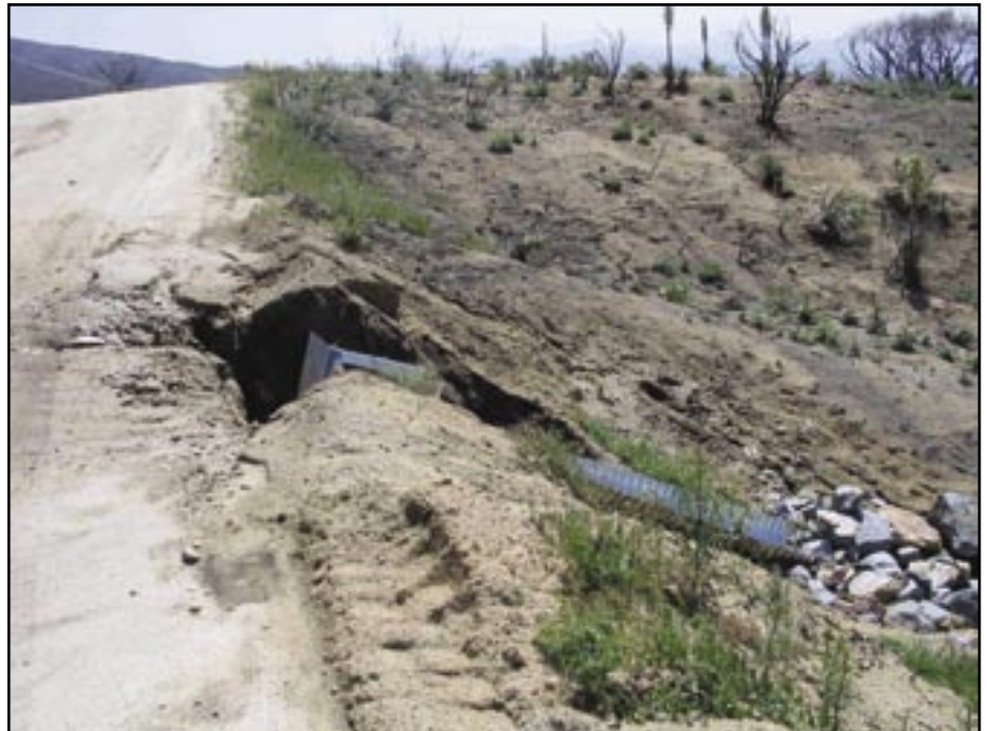
Figure 71—Failed metal roadside drain.
