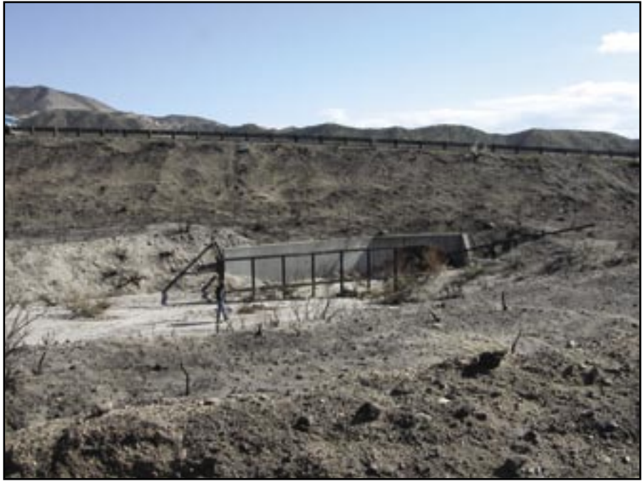
Figure 86—Large debris deflector on crossing below a major interstate.
