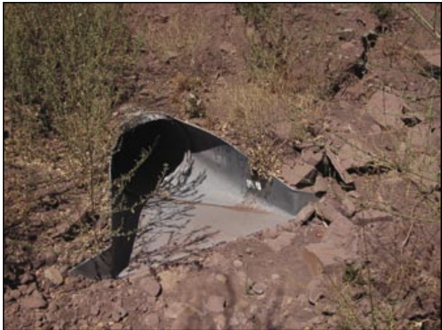
Figure 78—Metal end sections are attached to culvert inlets to improve the hydraulic efficiency and reduce the potential for plugging.
