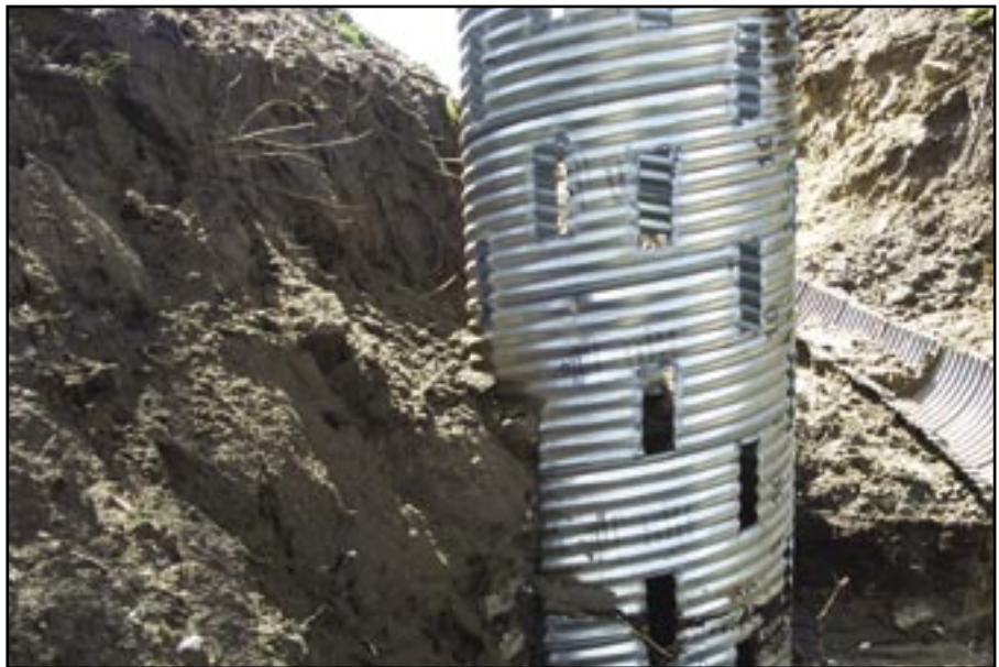
Figure 92—Ensure the openings on the riser are sized to allow water to flow freely into the structure. Small openings can plug with fine detritus.
