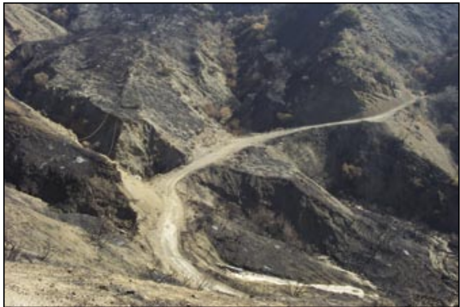
Figure 93—Removing accumulated sediment to ensure culvert capacity prior to seasonal storms can reduce the risk to the transportation infrastructure.
