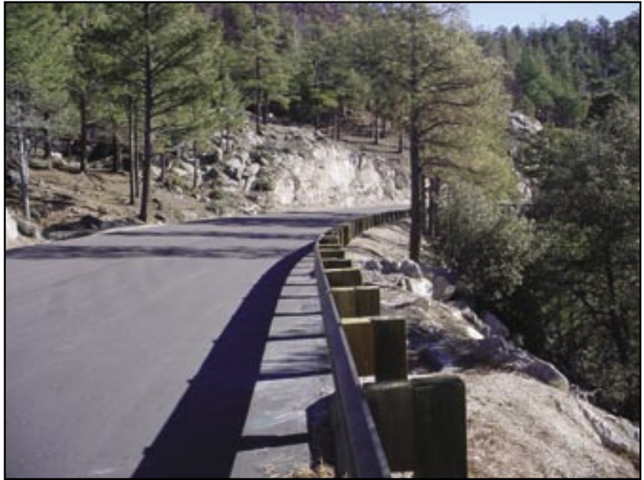
Figure 74—Imbricated rock level spreader used by FHWA in areas that burn often and control of water on the fillslope is critical.
