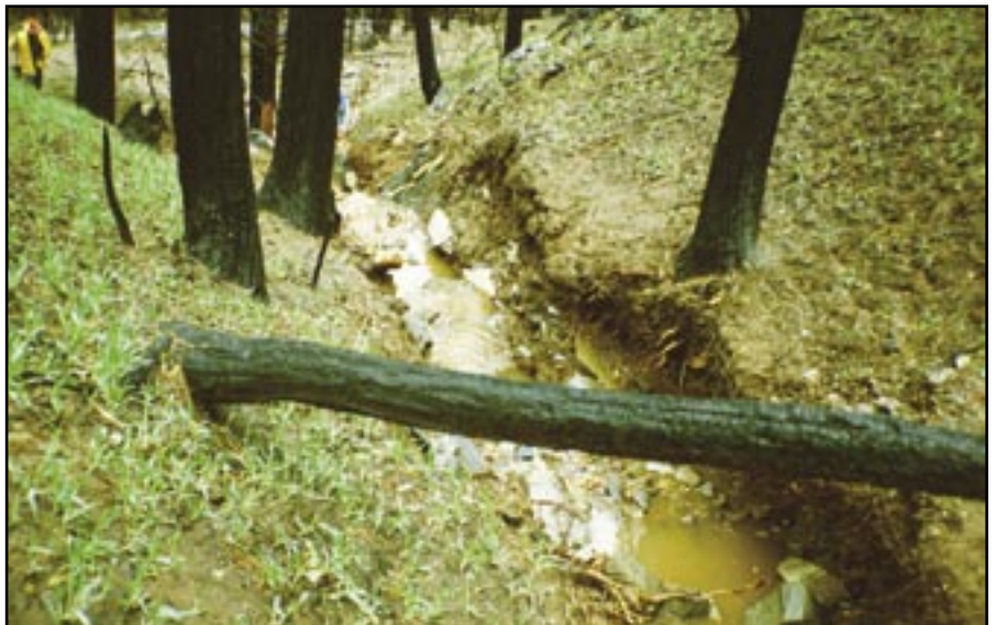
Figure 44—Seeded area is prone to accelerated erosion during the first year.
