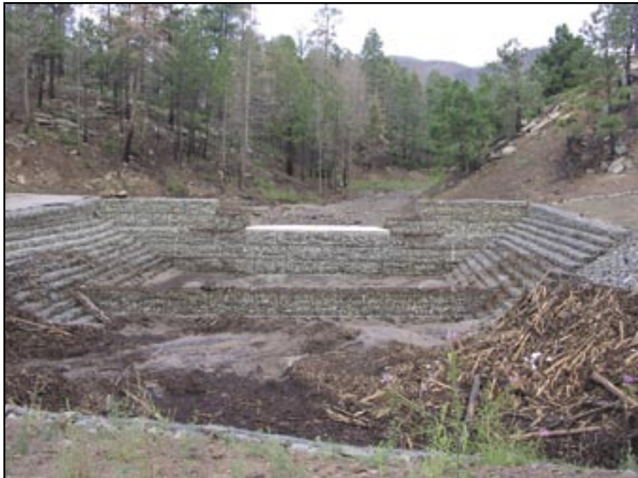
Figure 62—Large debris basins may be constructed where there are high values at risk.
