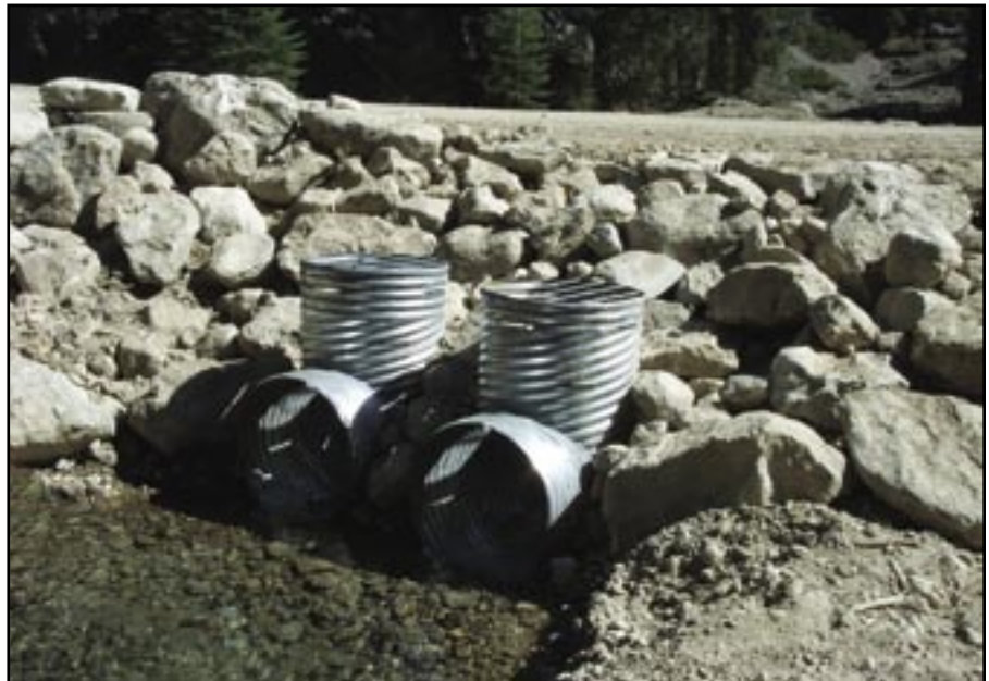
Figure 80—This culvert was modified with two culverts and risers to handle increased flows and potential woody debris.
